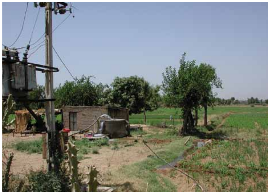
Power for groundwater pumping in Gujarat
